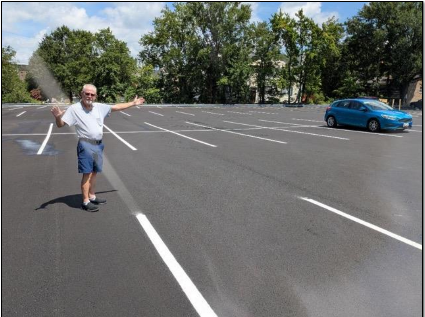
Ken Hall, Post 136 parking lot resurfacing project coordinator, said the project ensured that handicapped parking spaces received highly visible graphic signage and space markers. (Photos by Butch Hicks)
